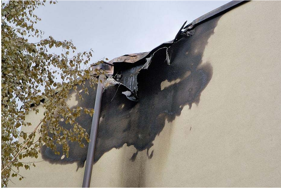
Fig. 5: Point of impact on the north-west side of the building at Roggenburgstrasse 15
